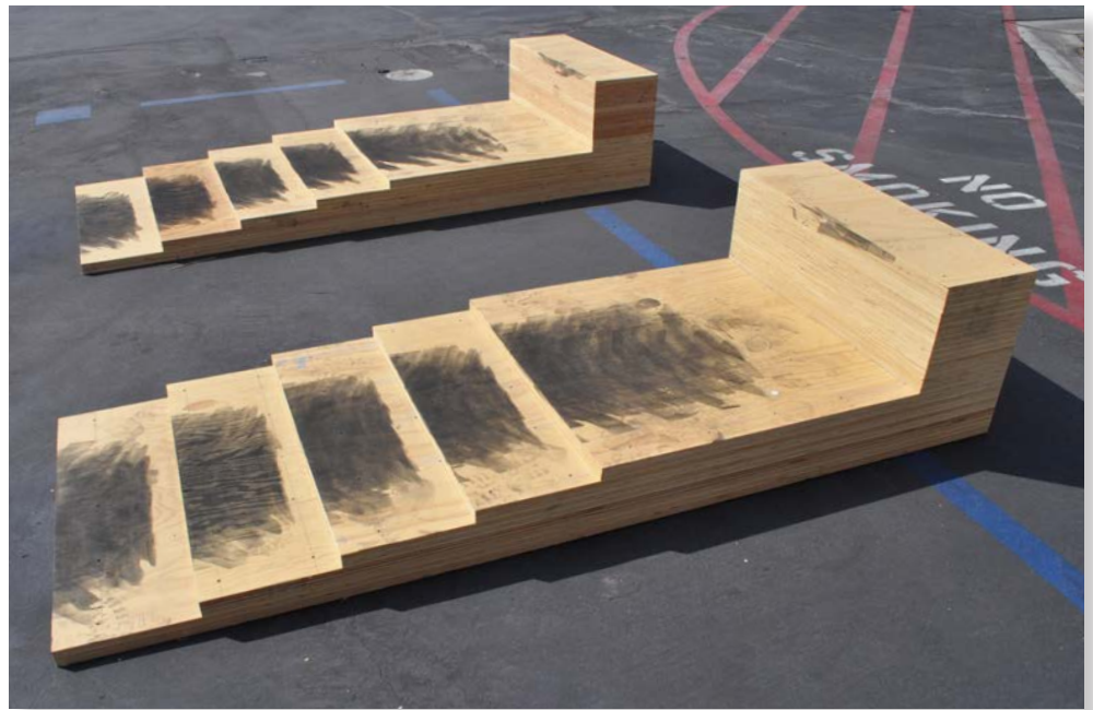
Figure 1.7. Cribbing blocks constructed for a boom lift. Scissor lifts cannot be leveled using cribbing.
