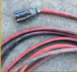
Damaged extension cord.
