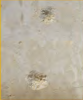
Spalling is the deterioration of concrete or brick due to age, wear, or a tool misfire. Spalled areas are not strong enough to hold a fastener.
