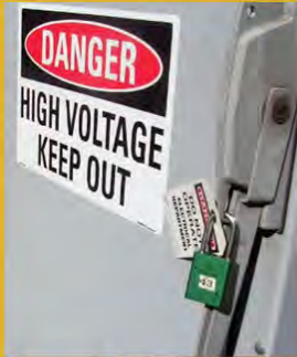
A lock and a tag on an electrical panel.
